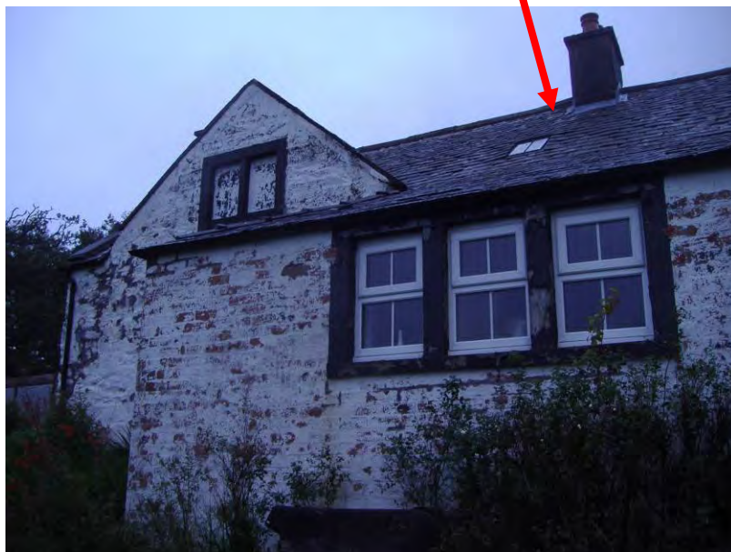
Photograph 2 – 28.09.2011. One Soprano pipistrelle emerged from below the slates to the east side of the chimney.
