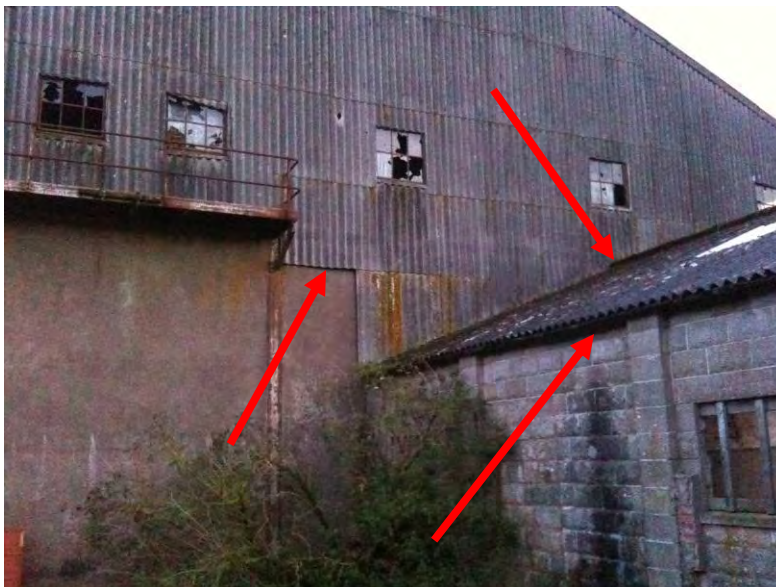
Photograph 1 – 21-22.09.2011. Three roost locations on the south-facing end of the large garage building, and the small stone shed attached to the south end of the garage. Note: the roost point indicated at the apex of the small stone shed is inside the shed
